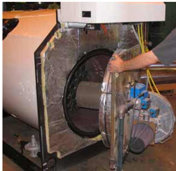
Figure B6-4. Burner maintenance
