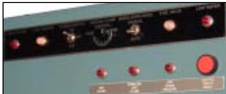
Figure 1-11 Control Panel Closed
